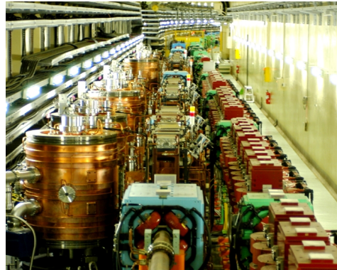
Figure 5: Many large ARES cavities (cylindrical shape lined up on the left) were installed in wide and long straight sections of TRISTAN.
