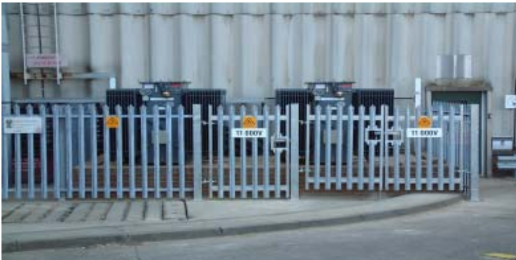
The new outdoor transformer bay showing two of the four 1.5MVA transformers
