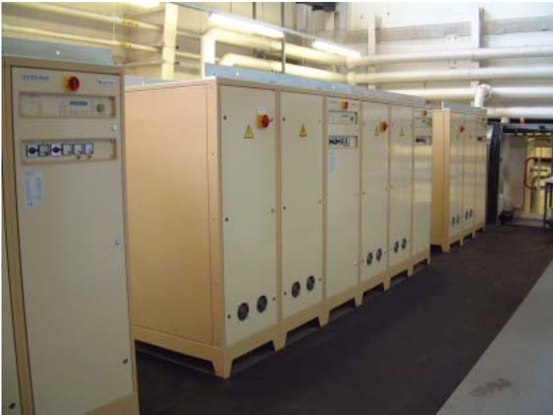
Hall 2 platform showing the four LVPS for the Bias systems.
