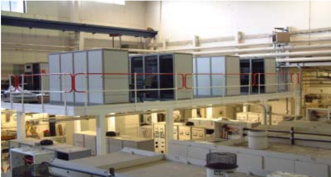
Hall 2 platform with racks for the HPD power supplies and controls
