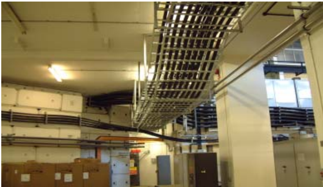
The sixteen, 4-core aluminium cables that run from the Bias Regulators to the cavities.
