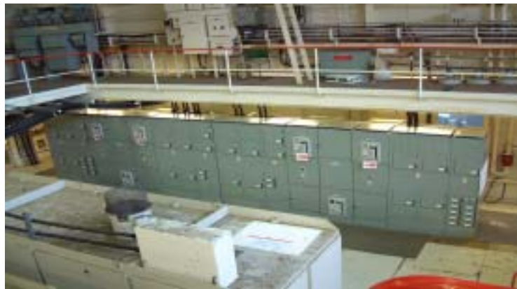
New 415V distribution board in Hall 2 (R5.4)
