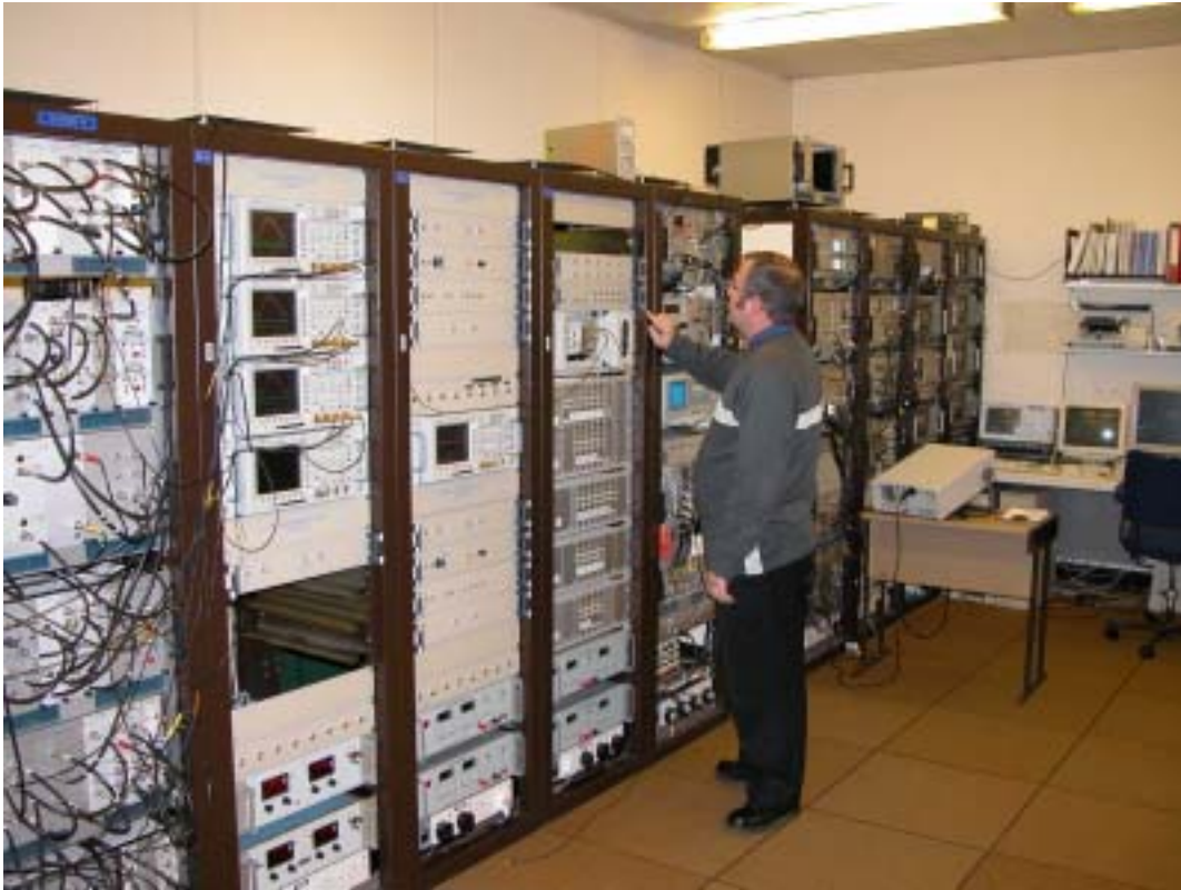
LPRF rack layout adjacent to the main control room
