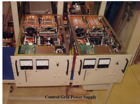
Figure 11: Grid power supplies.
