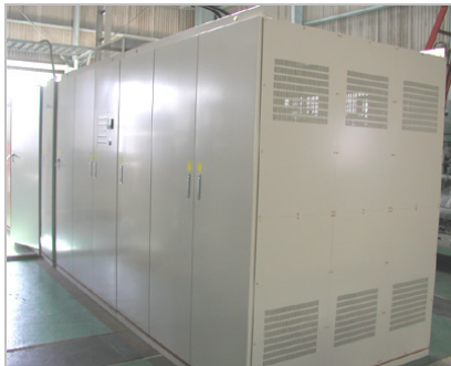
Figure 2: Power supplies for rf amplifier.
